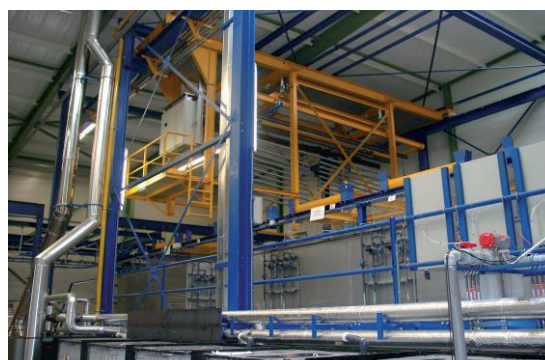
Trevelling crane for KTL coating plant
