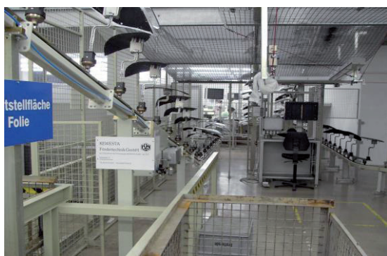
Inverted overhead conveyor 90NnV
